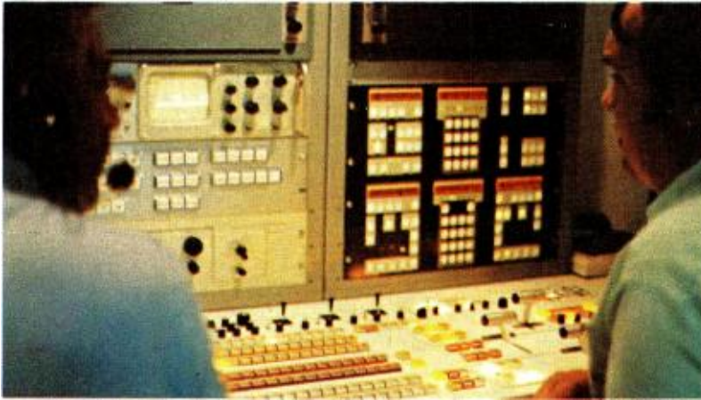
In Production Control at TV-30, the AE-600 remote editing control panels are rack-mounted above the video switcher.
