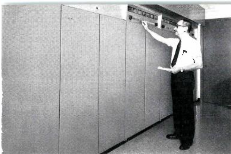
TV-52's 110 kW transmitter, TTU-110, is checked by Transmitter Supervisor Max Thomas.
