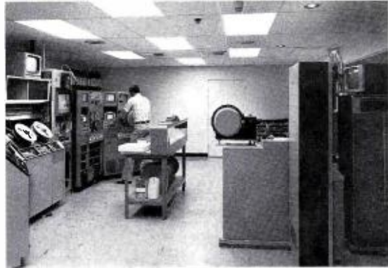
Video tape and telecine systems are located in a separate humidity-controlled room. TR-600A tape machines handle most of the subscription television programming.
